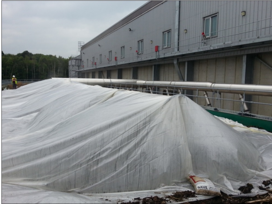
Plate 6 Sampling of the open biofilter at UOL05
