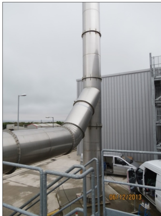
Plate 1 Outlet stack from biofilter at Site UOL01
