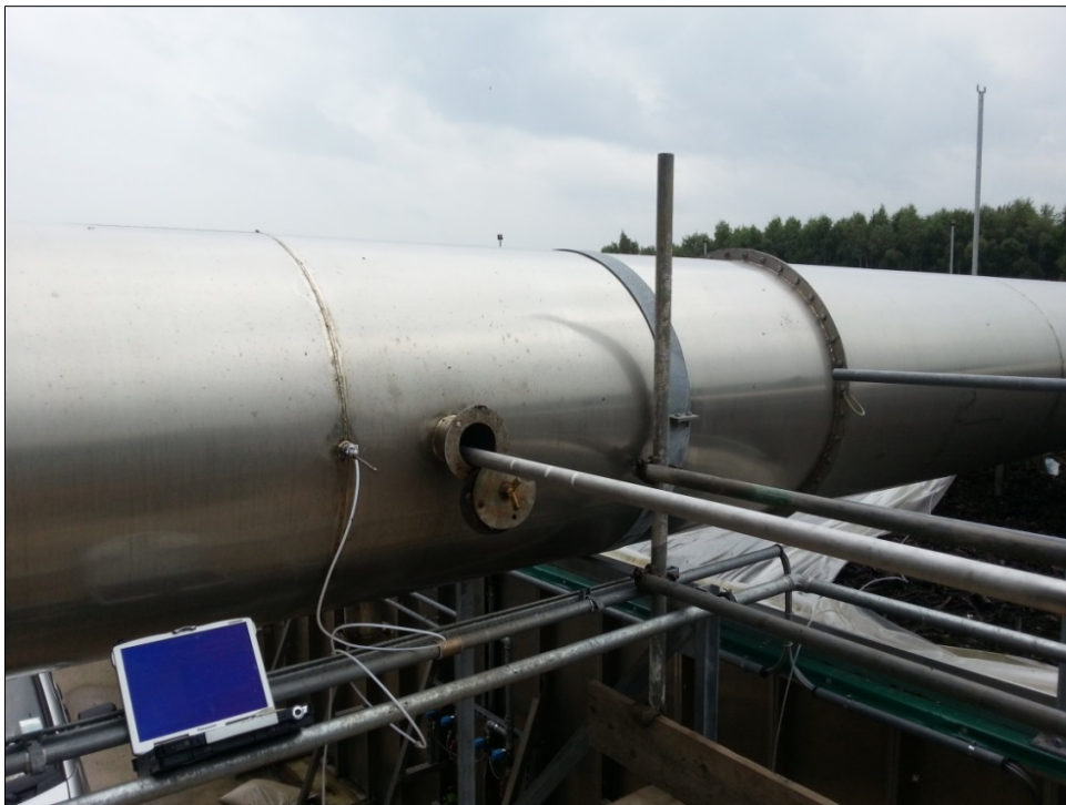
Plate 5 Sampling from the inlet duct to the open biofilter at UOL05
