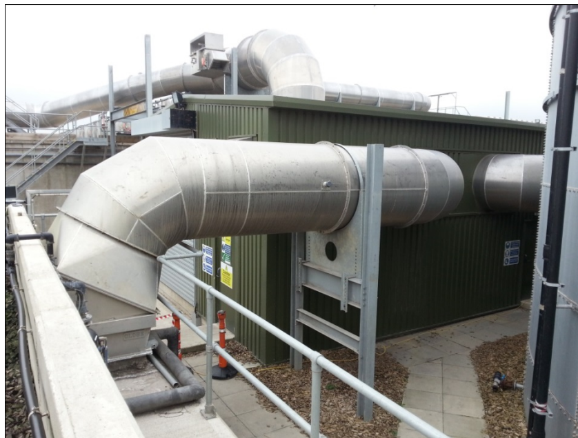
Plate 10 The biofilter inlet duct at UOL07
