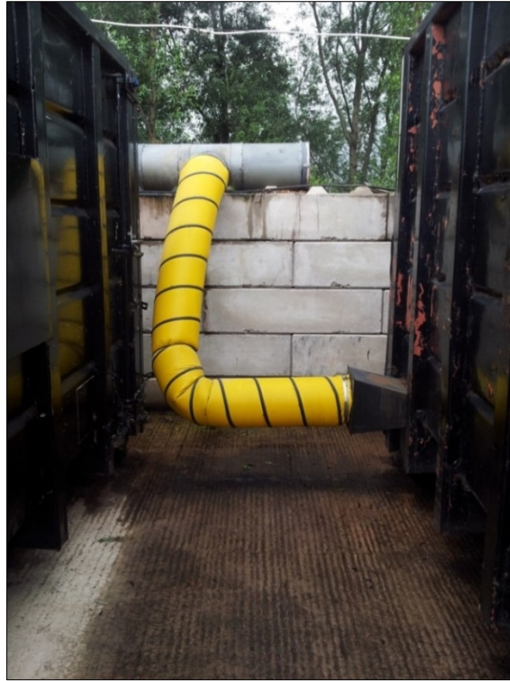
Plate 8 Inlet duct to biofilter 4 at UOL06
