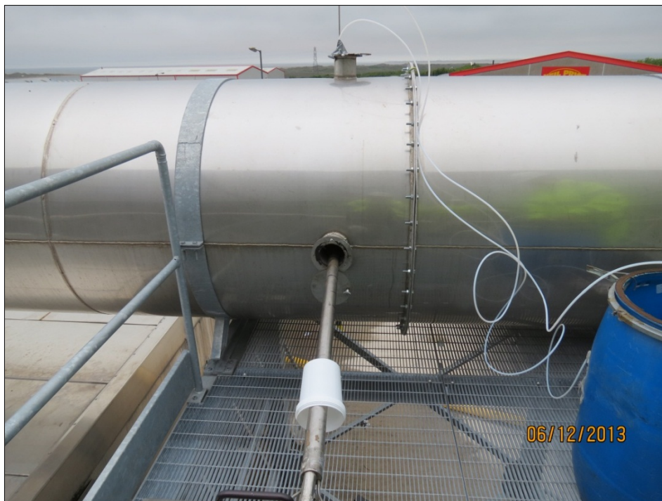
Plate 3 Sampling from the biofilter outlet duct at Site UOL01
