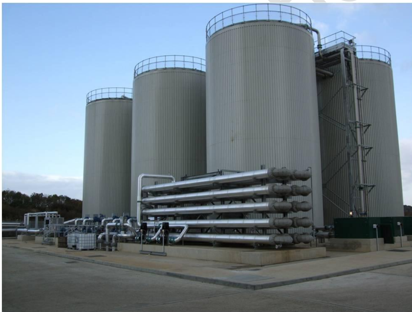
Figure 3 Enhanced enzymic hydrolysis reactors at the Great Billings sludge treatment centre operated by Anglian Water and achieving a 6-log removal of E. coli
